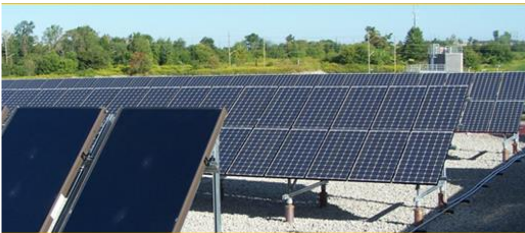
Figure 19. Photovoltaic solar panels at the Ajax Operations Centre
